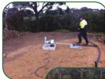
These 3 pictures show the aeration system being installed, and then in working order.
